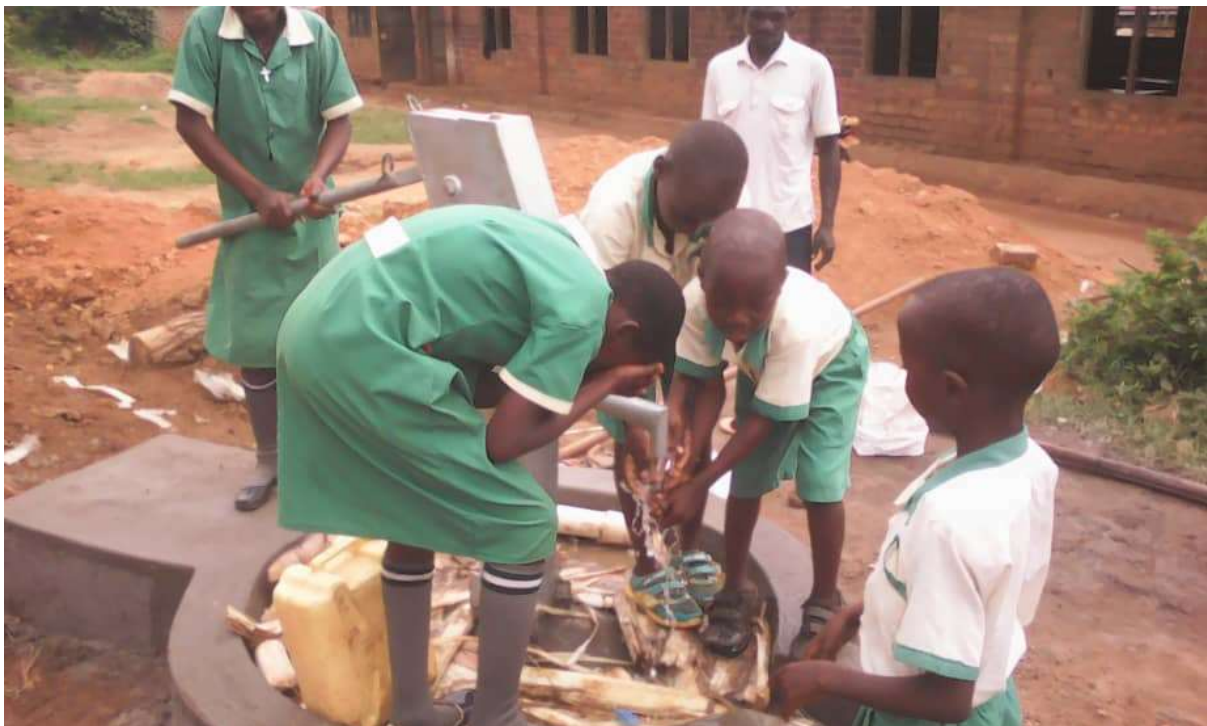
Figure 27: Nalumansi primary school pupils pumping water from the newly constructed shallow well. Photo by JEEP.
