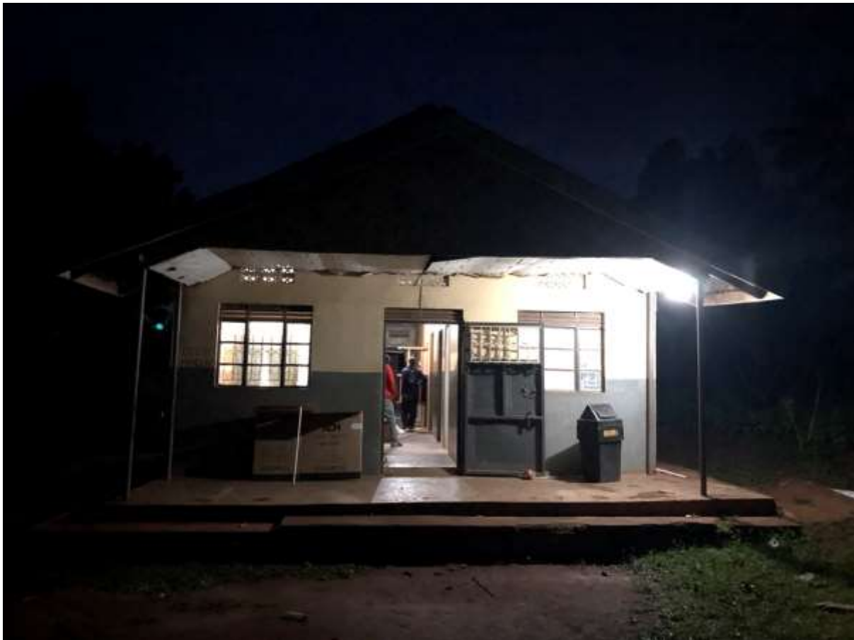
Figure 18: Kafumu Health Centre II after the installations. Photo by JEEP.
